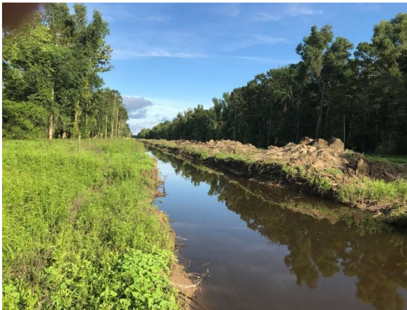
Figure 2. A typical channel after excavation and cypress tree removal. A low friction conduit.
