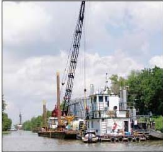
RAISON D'ETRE? — Oil and gas operations in full swing on Bayou Postillion. Activity began soon after the channel was deepened with state funds, ostensibly to improve water quality for fishermen. (Staff Photo by Sally Angelle)
